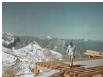
The heliport as a timber construction. A generator was installed inside to provide the team with essential electricity.
